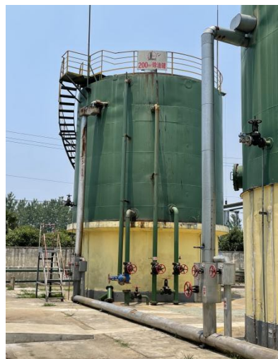
沙埕联合站除油罐
